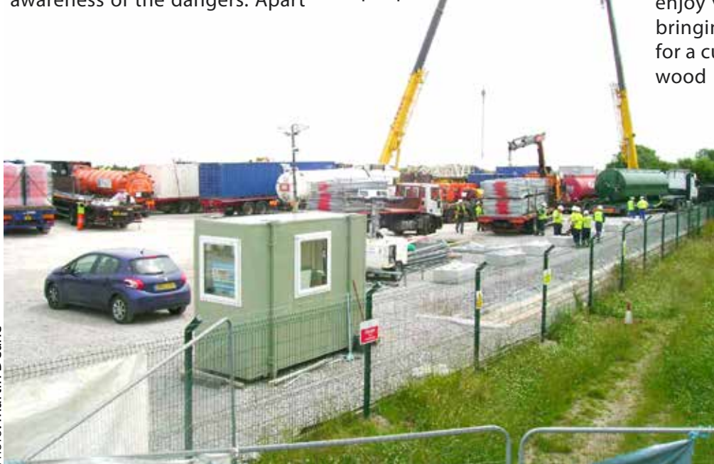
Vehicles arrive at the West Newton site to begin drilling. This is not the full extent of the equipment.
