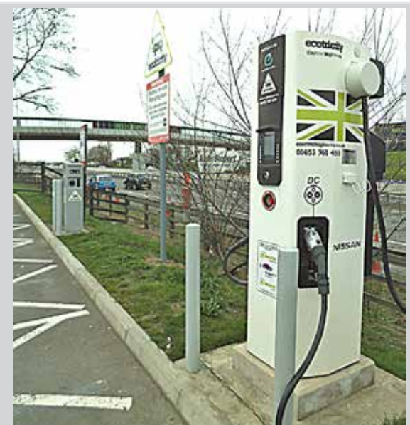
Electric car charge point: Woodall Services
